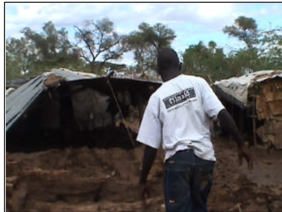
FilmAid staff member Okello Charles surveys the damage done to his house
